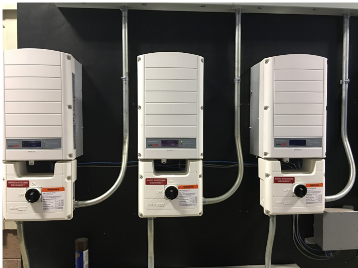
Inverter used to convert solar to useable power.
